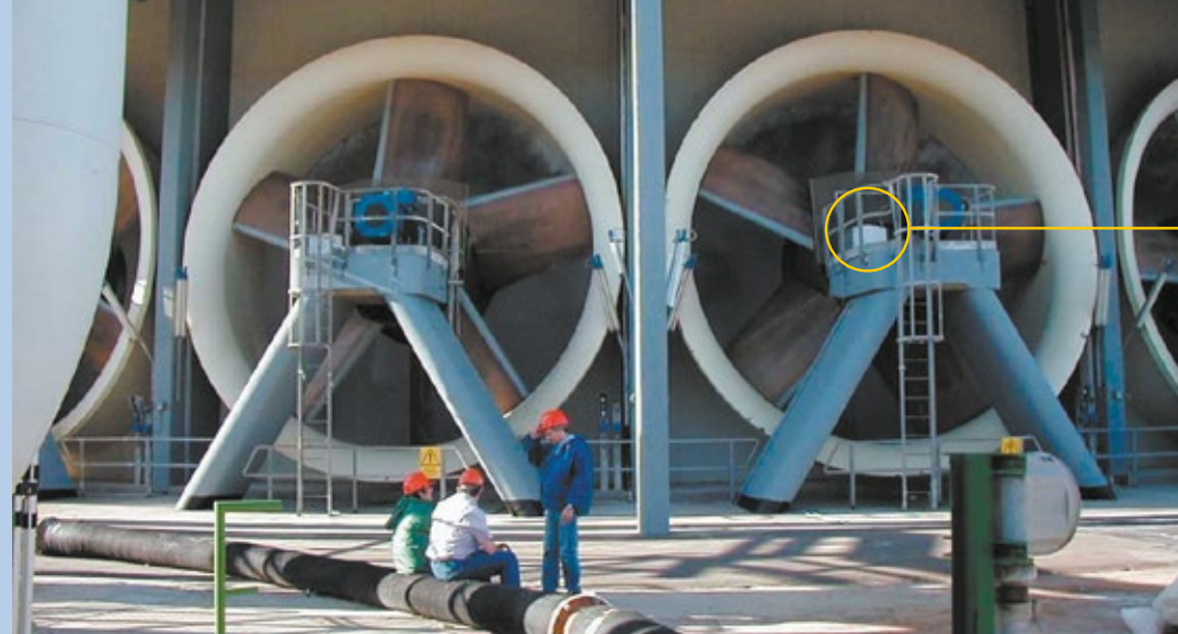
Fans in a Cooling Tower – Scholven, Germany
